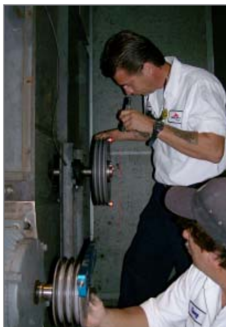
The photo above shows mis-aligned pulleys.
