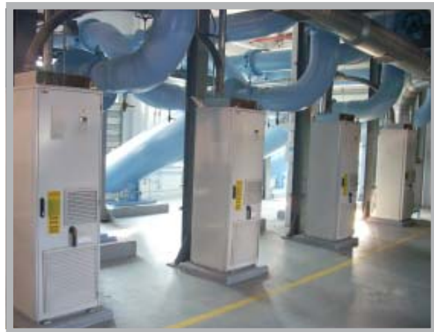
The Dam Neck Annex of NAS Oceana upgraded HVAC infrastructure in 36 buildings and decommissioned the central steam plant by implementing geothermal water source heat pumps. The entire project was funded through operational savings.
